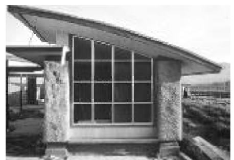
Figure 76: Real Goods Solar Living Center in Hopland, CA (top); detail of straw bale wall (bottom) (Daniel Smith & Associates)
