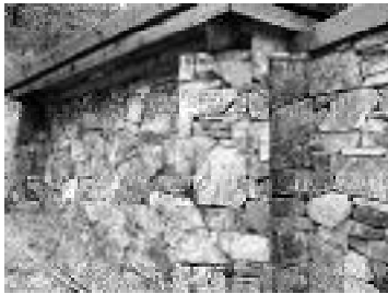
Figure 77: Trinity Springs bottling facility in Pine, Idaho (top; The Underground Water People) curves around the springhouse built from dry-stacked stone (bottom; Erik Barr).
