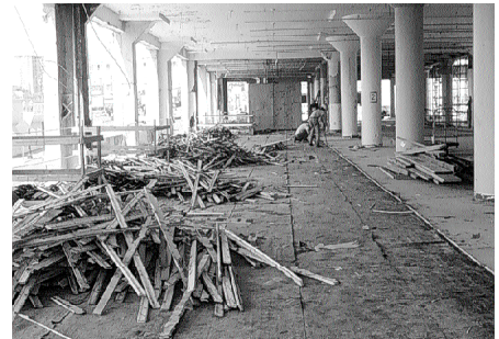
Figure 26: hardwood flooring salvaged by a local reuse business (Metro Portland Solid Waste)
