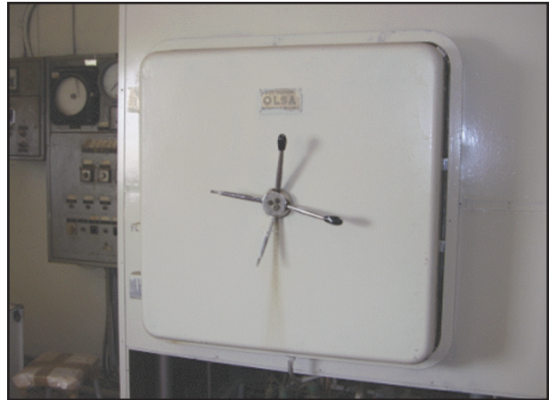
Autoclave with control panel.
