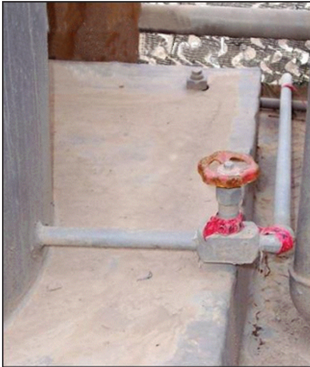
Figure 7. Outlet valve and pipe on the reactor vessel of trailer 1.
