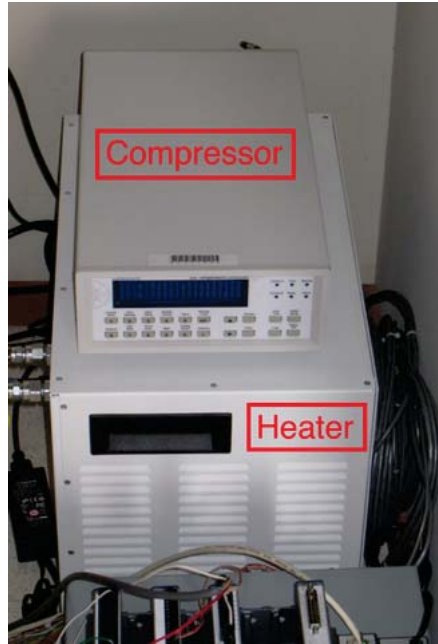
Figure 13: Heater and Compressor. The power supply box and control modules are visible in the foreground.
