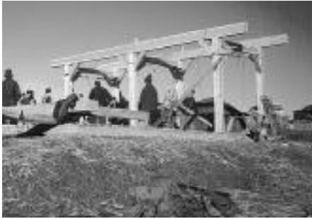
Figure 44: Raising the timber framework of a studio built by Keith Smith, Moscow, Idaho
