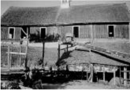
Figure 41: Conservative disassembly of Pickering Barns using a snorkel lift, Issaquah, Washington (KPG, Inc.)
