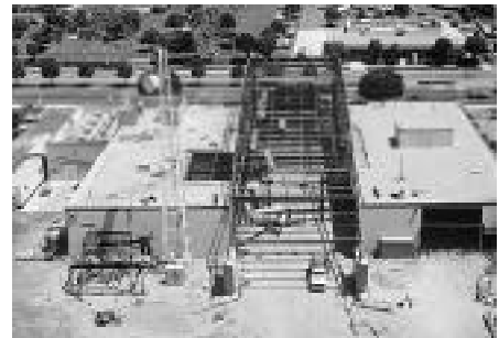
Energy Resource Center in Downey, California: Figure 32 (top) illustrates the original building, while Figure 33 shows the “open-heart surgery” (Southern California Gas Company)
