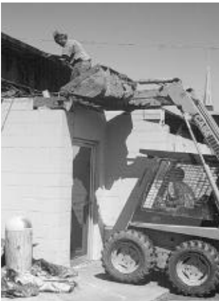
Figure 42: Wasankari Building Recyclers salvaging tongue and groove roof deck of the old Bowl-A-Rama, Moscow, Idaho
