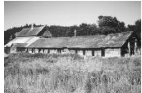
Figure 35: Pickering Barns showing dilapidated state of original building (KPG, Inc.)
