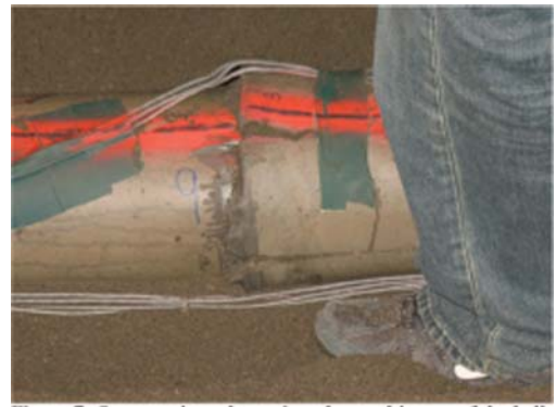
Figure 7. Compressive telescoping observed in one of the bell-and-spigot joints adjacent to the fault plane.
