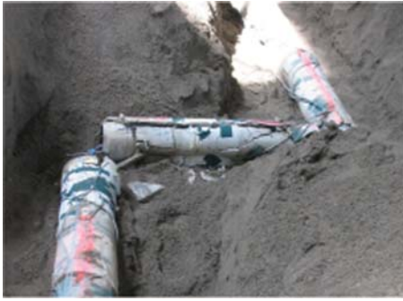
Figure 8. Pipeline deformation observed near the fault. Note that the fault plane ran through the middle of the pipe segment shown in the center of the figure.
