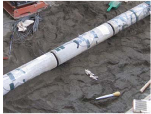
Figure 4. Assembled pipeline segments prior to joint grouting. Grout was poured in the annular space shown at each joint location.
